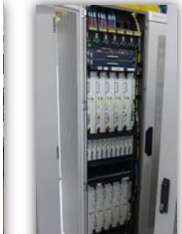
2 DTN-X racks like this one were used at each end
